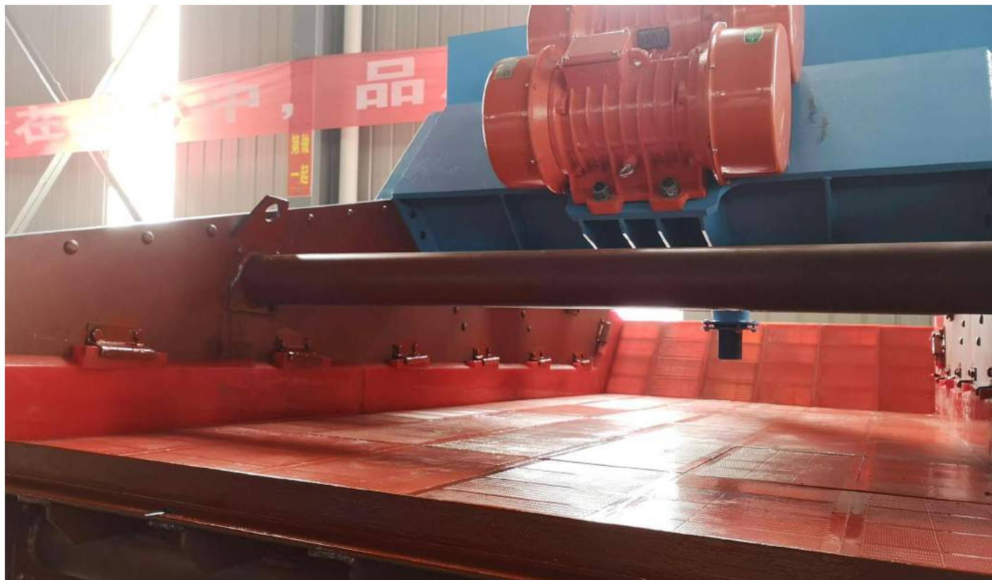
c. Solid waste dry discharge – dry discharge and dry heap treatment of solid waste in tail water
